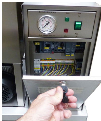
Fig. 5 Steam generator front cover
