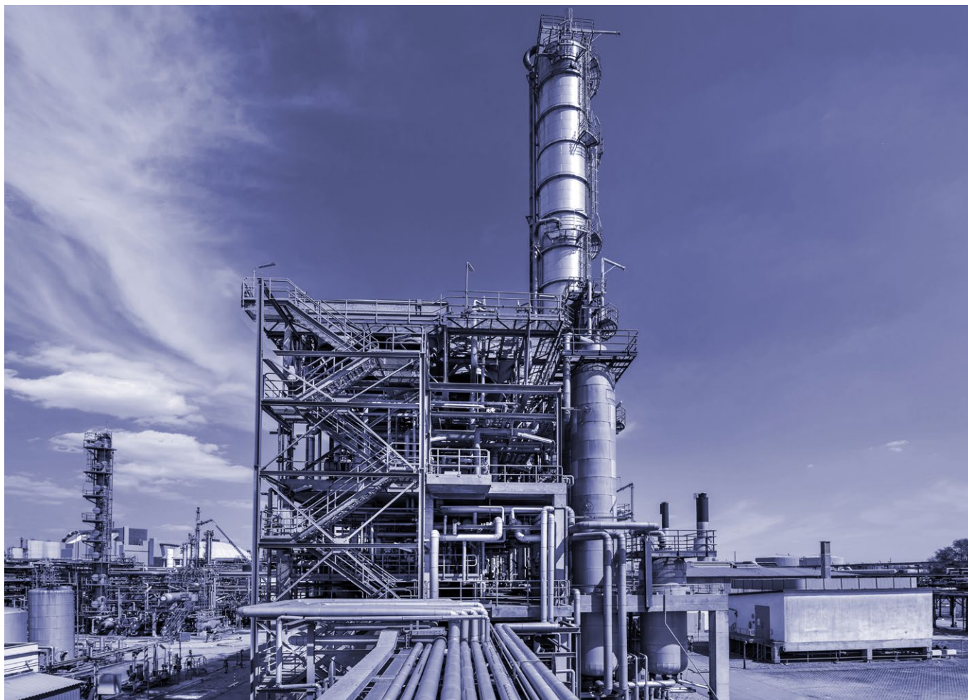
Holborn refinery crude oil distillation plant.
