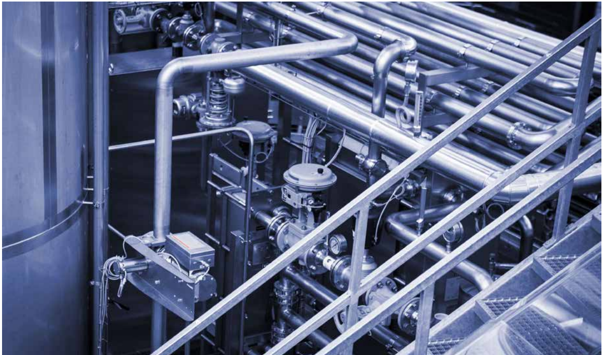
Process monitoring: The Beer Monitor from Anton Paar analyzes the beer during production.
